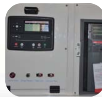
Control Panel & MCB
